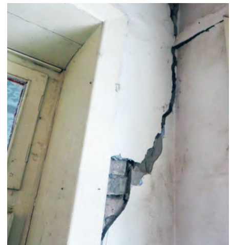
Structural damage on the interior wall of a school in Balkh Province. (SIGAR photo)
